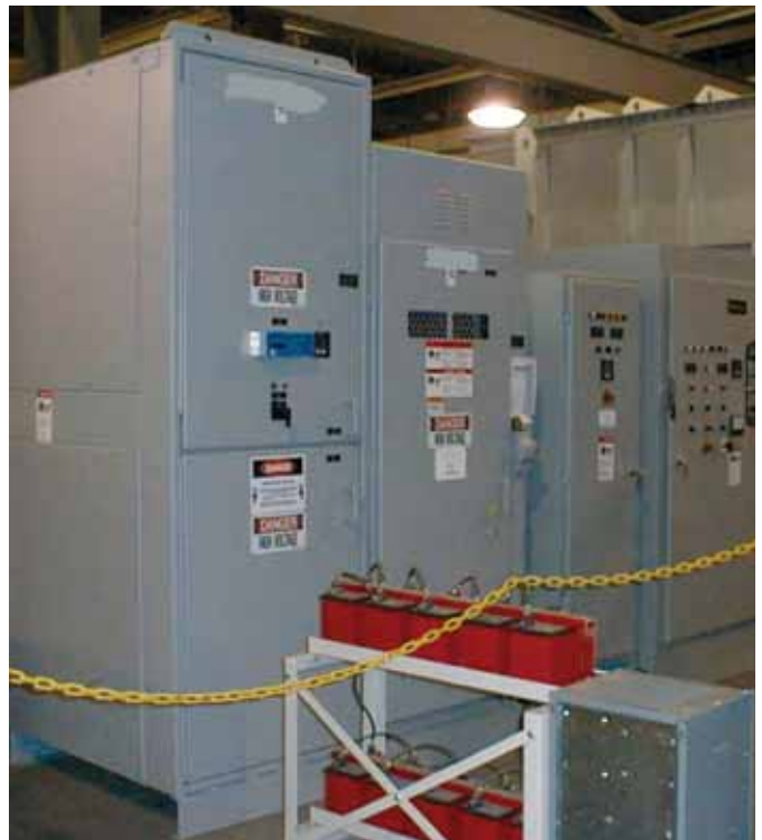
15 KA @ 380 VDC Chlorine Supply
