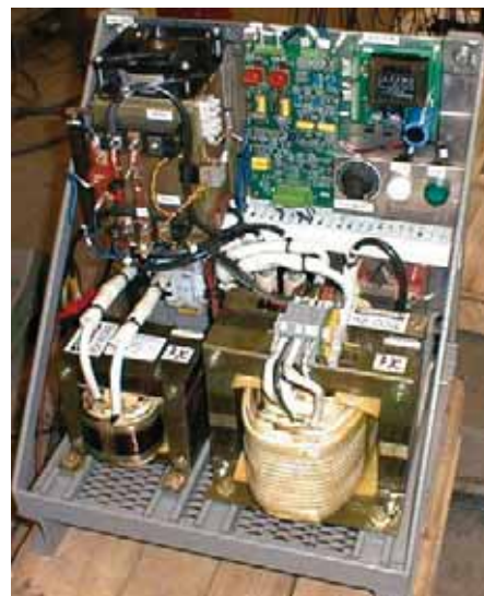
DC Supply with Reactor
