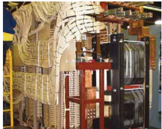
16 MVA Rectifier Core & Coil
