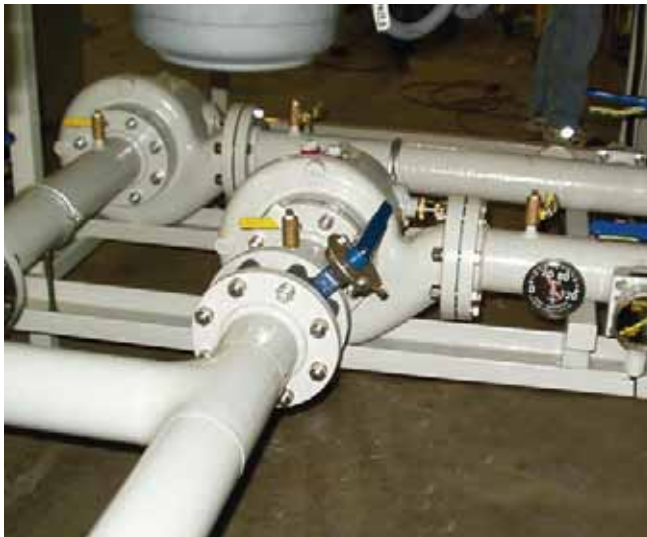
Dual Pump Cooling for Oil-Filled Transformers
