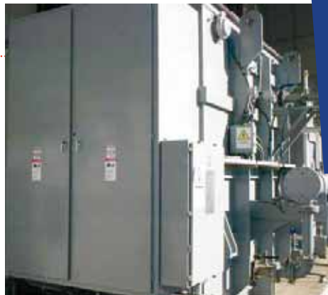
83 KA @ 266 VDC Chlorate 12 Pulse Transformer/Rectifier
