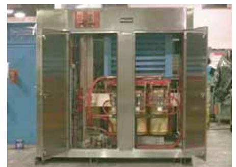
Nema 4x DC Power Supply
