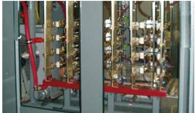
40 KA @ 200 VDC DC Power Supply, installed in Thailand for Zinc.
