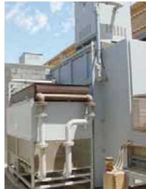
12 MVA Rectifier-Transformer with Oil to Air Cooling
