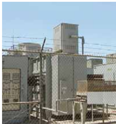
40 KAC @ 200 VDC Power Supply for Zinc Extraction
