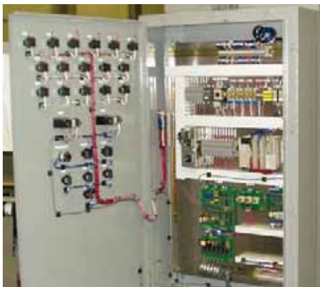
Cathodic Protection DC Power Supply
