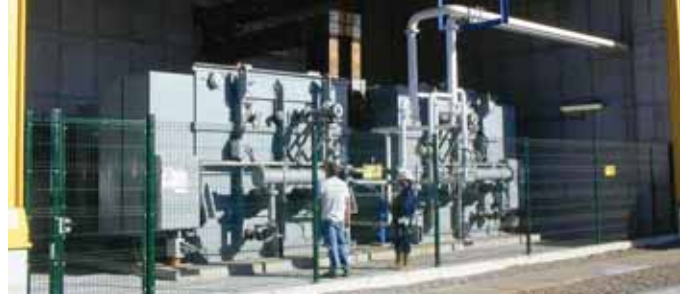
83 KA 12 pulse Transformer/Rectifier Line-up
