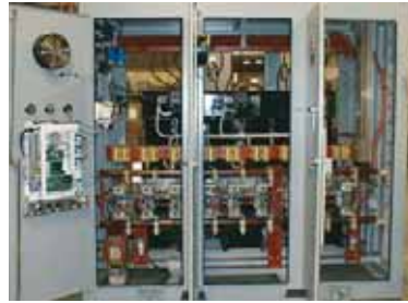
High Power Water-Cooled Reactor in Arc Furnace Supply
